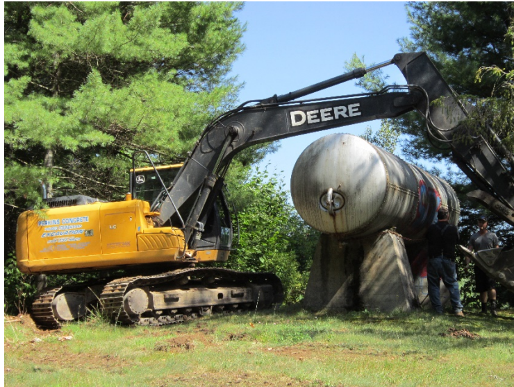
Photo of contractor rotating the rusted water tank at the Milton Mills Town Cemetery so water will be available for the first time in eight years.
