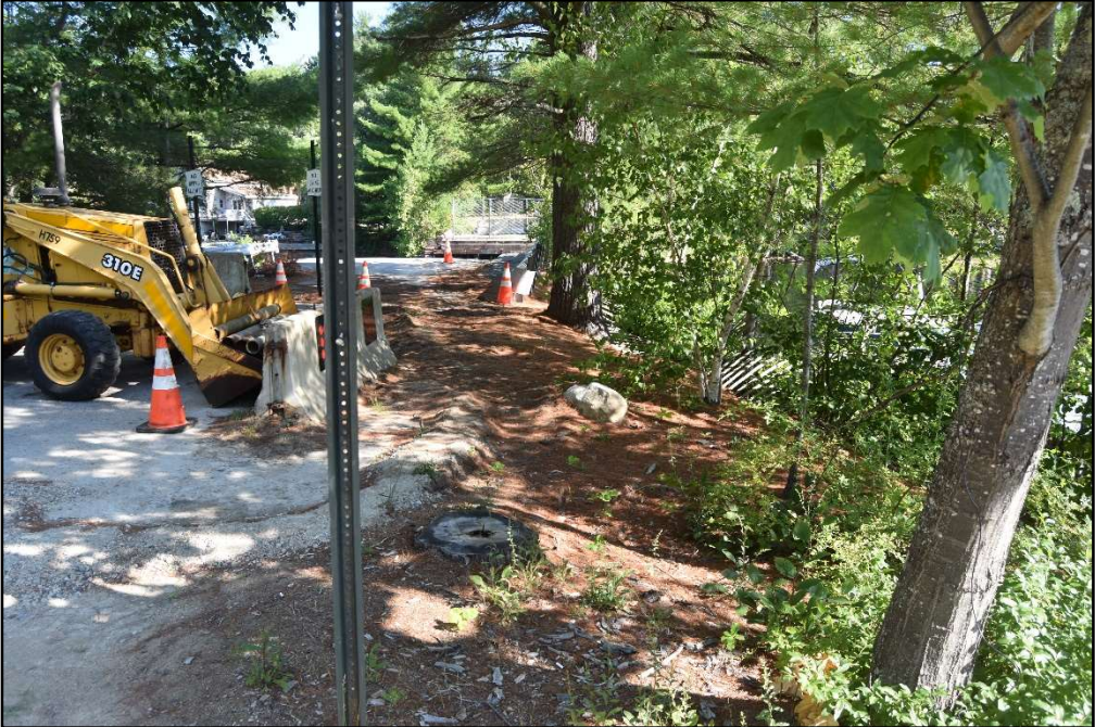
Figure 17. Steep fill slope along the eastern road edge near the bridge, view northwest.
